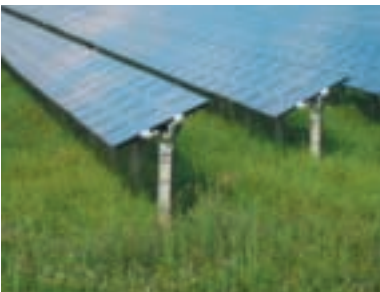
Photo-voltaic Panel Arrays
